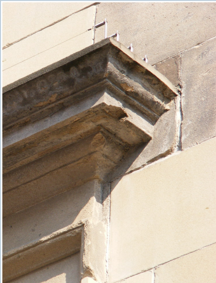
Discreet sprung wires are attached to the top surface of this cornice to deter birds. Miller Street, Glasgow.
